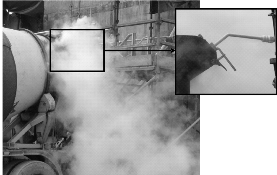
Figure 6.6 The use of liquid nitrogen to cool concrete on site immediately before placing
